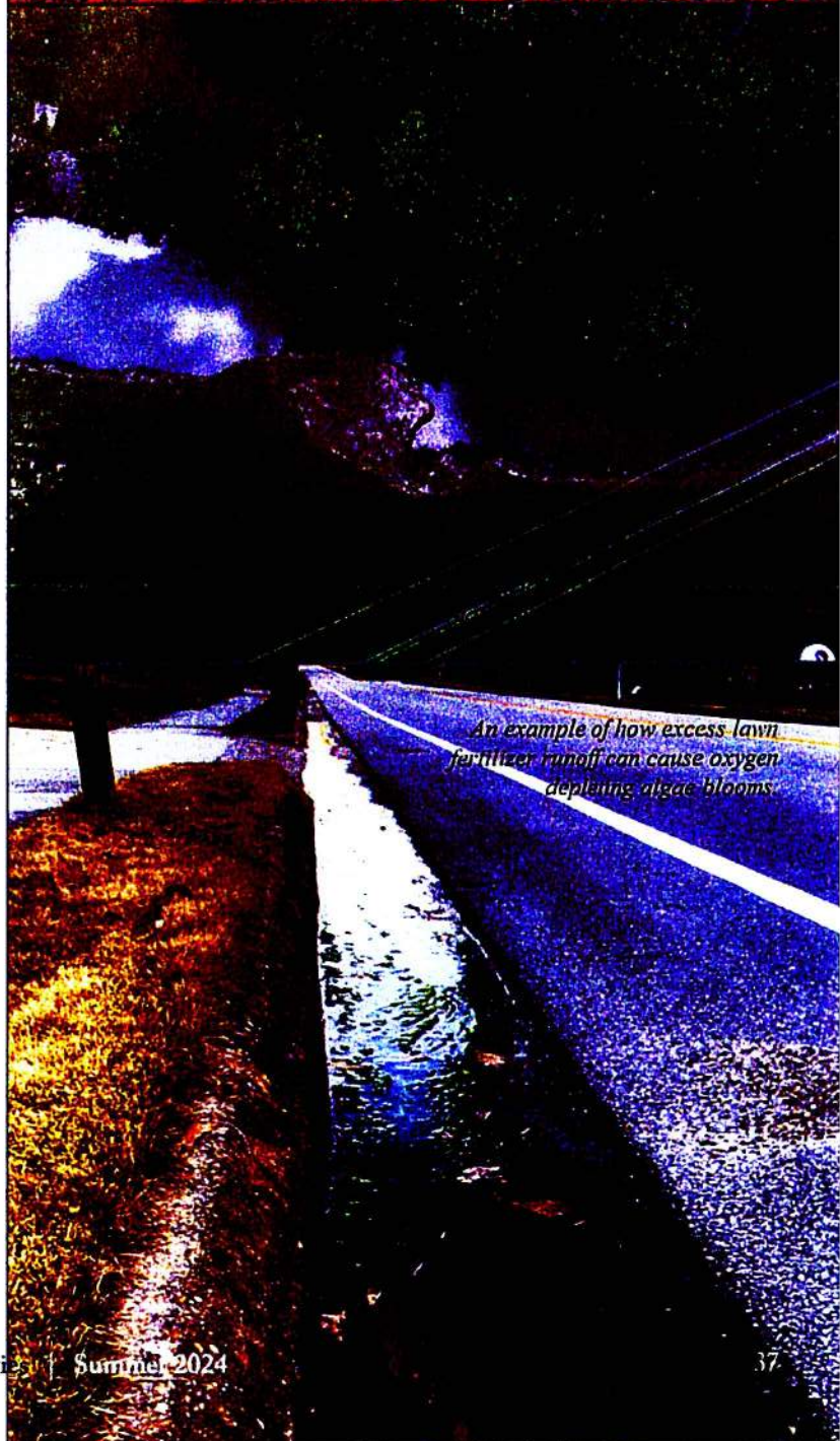
A construction site in need of erosion and sediment control. In a rain event, this sediment will be washed into waterways.
